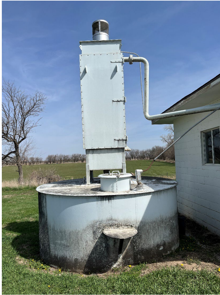
Figure 9 - City of Randolph Aerator and Detention Tank
